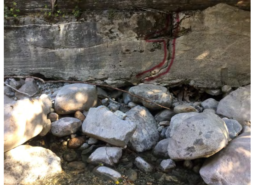
Scour under CIP extends 600mm in places
