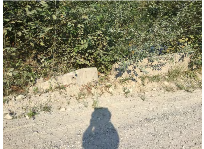
Bullnose not connected at upstream right approach
