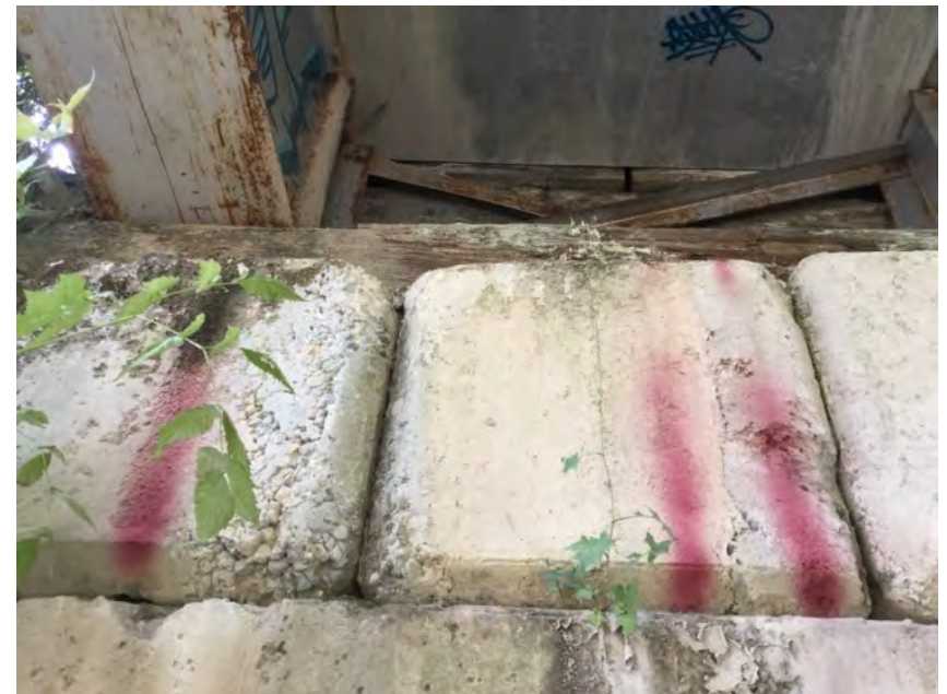
Lock block condition
