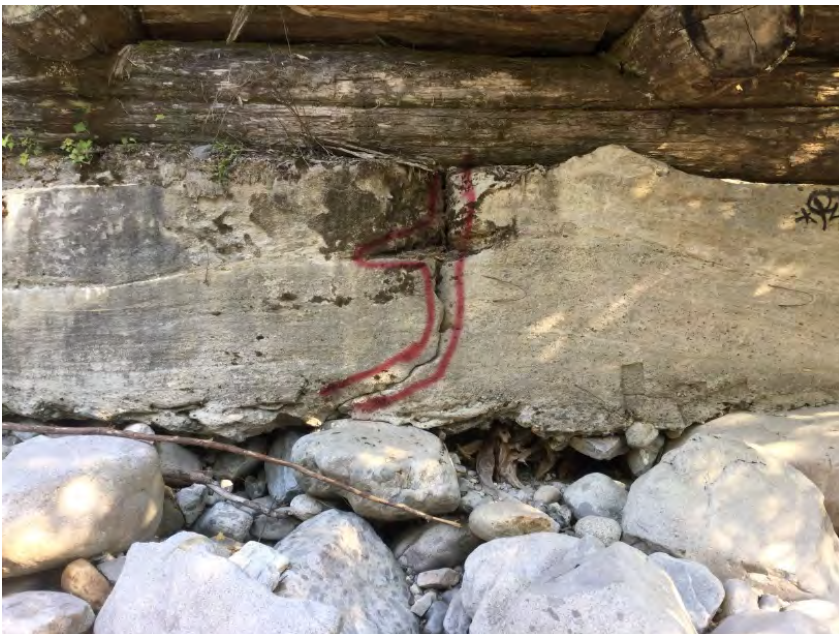
Vertical crack in CIP
