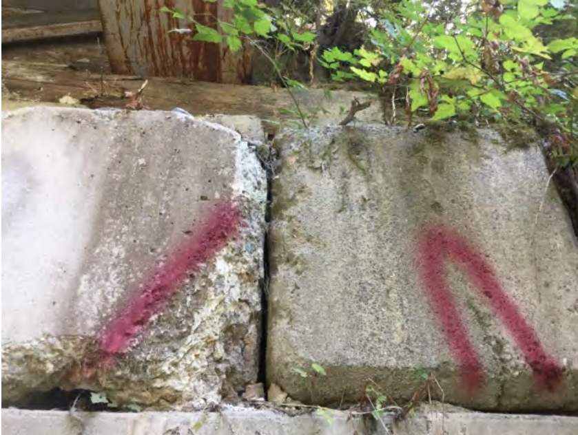
Lock block condition
